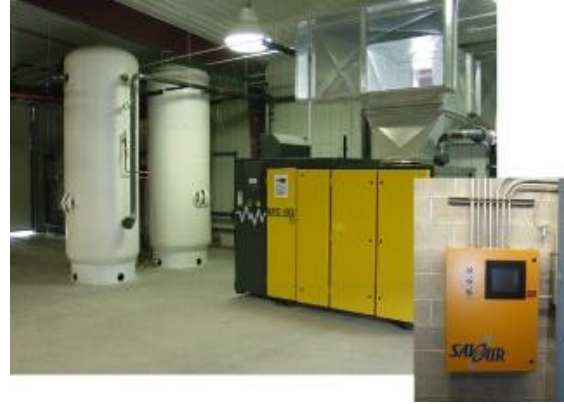
Figure 3. Luzenac Compressor Room
